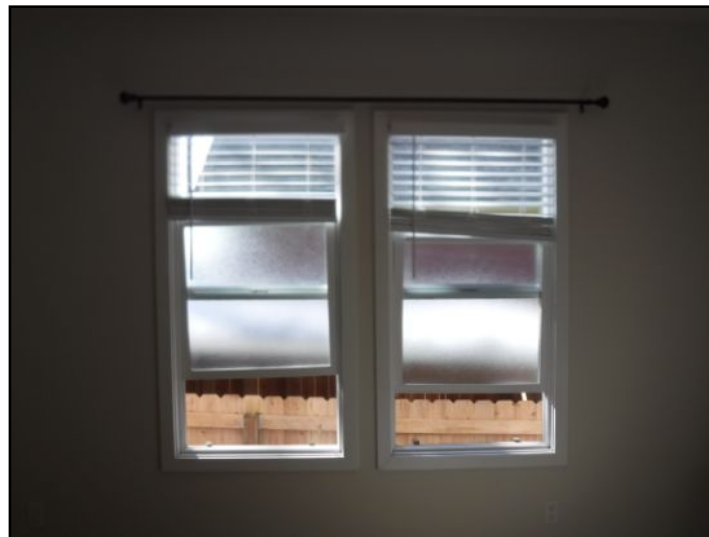
Both Windows: Counterbalance system is damaged, missing, operates poorly or not operative. Recommend corrections to restore function.
