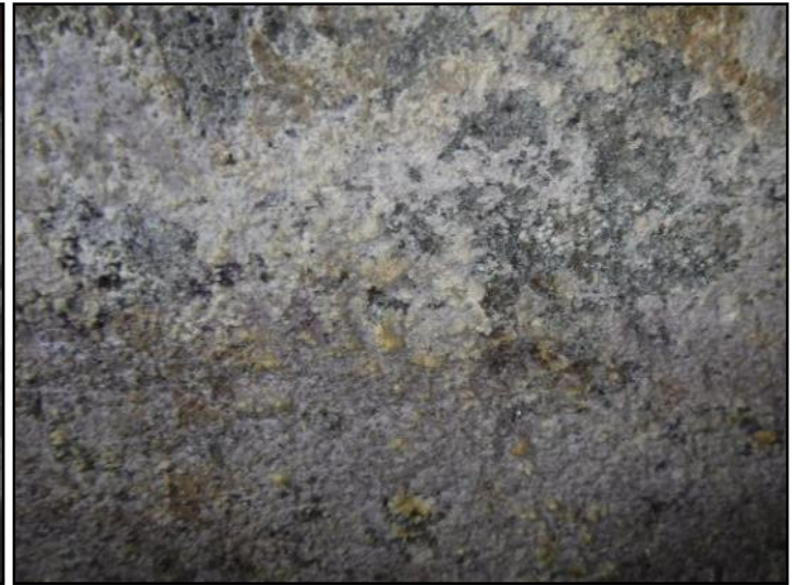
Efflorescence observed; this is a mineral deposit left behind from previous exterior water infiltration. Consult with drainage experts for best applications of drainage systems for outside the foundation perimeter and within the perimeter.
