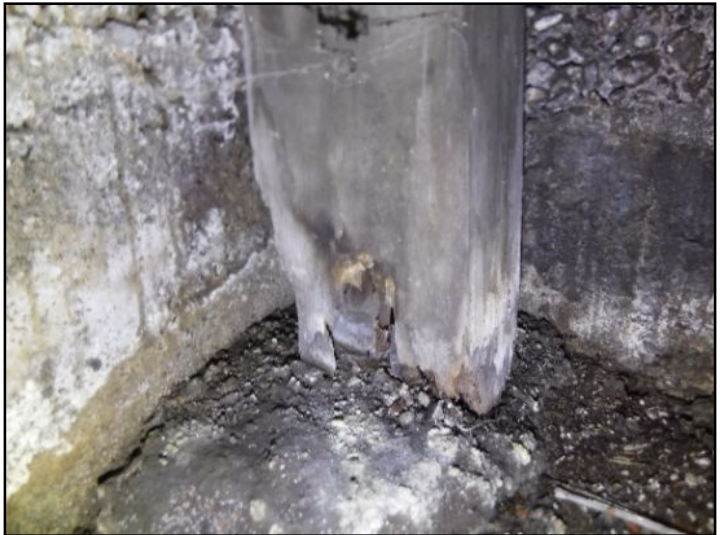
Water damage / decay noted at the base of several posts below basement stairs. Corrections by a licensed contractor is recommended.
