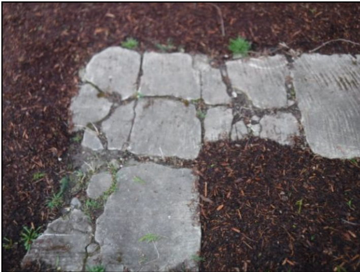
Walkway - Moderate to significant cracking / surface damage noted. Recommend consulting with concrete specialist to determine best course of action.
