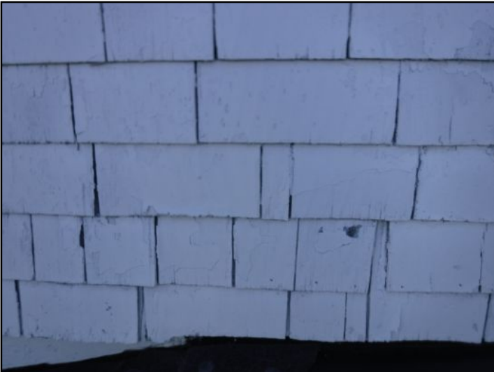
Older siding is intact, but shows some signs of aging. Monitor for wear. Repair cracks, gaps or holes as needed. Treat surfaces with stain or paint as needed to protect against siding damage and structure against the elements.
