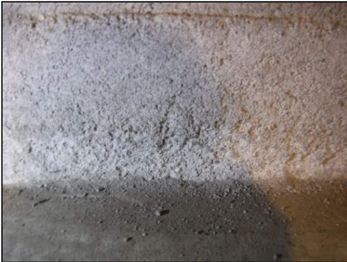
Spalling / deterioration noted on concrete foundation walls. It is recommended to have a foundation specialist evaluate the foundation walls and provide services to prevent further spalling / deterioration.
