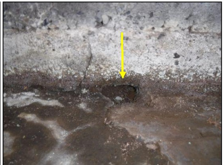
Gaps / eroded areas noted below foundation walls in some locations. It is recommended to have a qualified professional back fill these areas and seal the openings to prevent further erosion.
