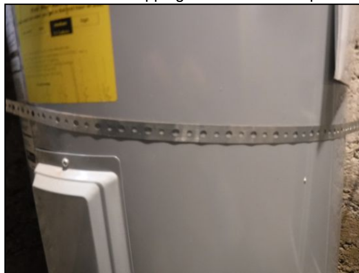
The water heater is strapped with plumbers tape. Recommend upgrading to Hot Water Heater strapping which is more capable of handling movement.
