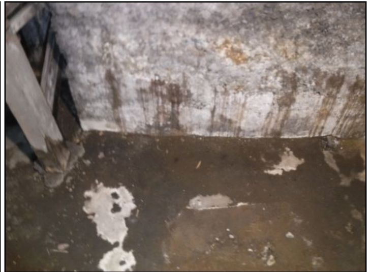
Moisture intrusion was observed numerous areas of the foundation. Moisture can create high humidity, mold & can damage stored items & finishing materials. Recommend a wet basement specialist review the foundation for correcting the water intrusion and advise as needed.
