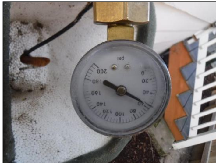
55 psi was the approximate pressure noted at exterior faucet
