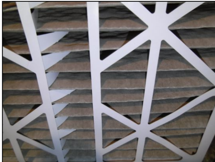
Furnace filter dirty. Needs replacement.
