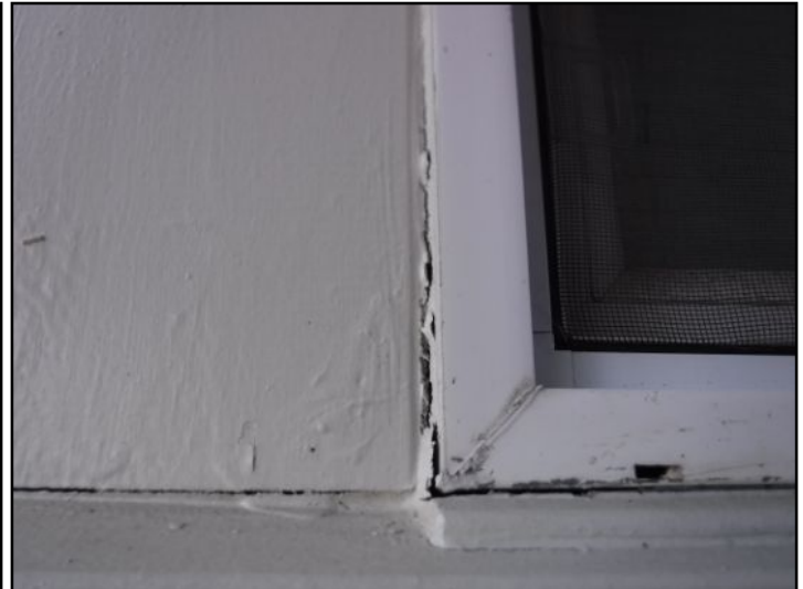
Caulking missing or damaged. Recommend correction by qualified professional to protect underlying materials from damage.
