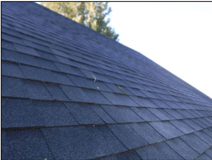
The asphalt shingles appeared to be in good condition with minimal wear
