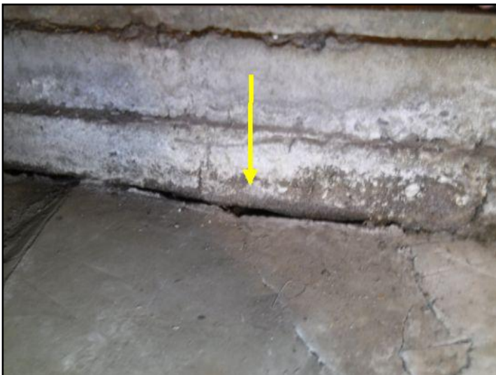
Gaps / eroded areas noted below foundation walls in some locations. It is recommended to have a qualified professional back fill these areas and seal the openings to prevent further erosion.
