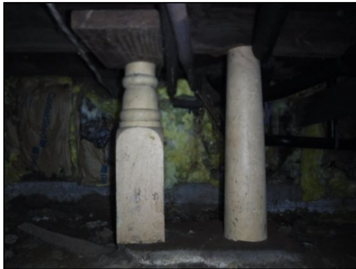
Interim support structures noted which are support devices which have been added to the foundation area to provide additional support in a specific area where it was needed.
