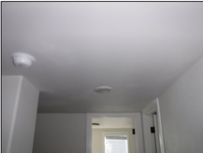
Small enclosed area above the ceiling on the upper level has no access point. Recommend installation of access point and evaluation with corrections as needed by a qualified professional.
