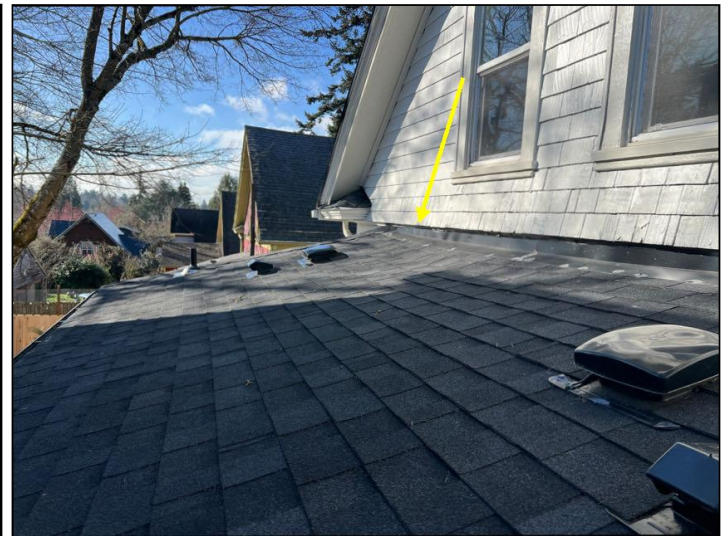
Lower level roof at rear of home: Areas of rooftop are sagging or bowing. Recommend evaluation and repairs as needed by qualified contractor.
