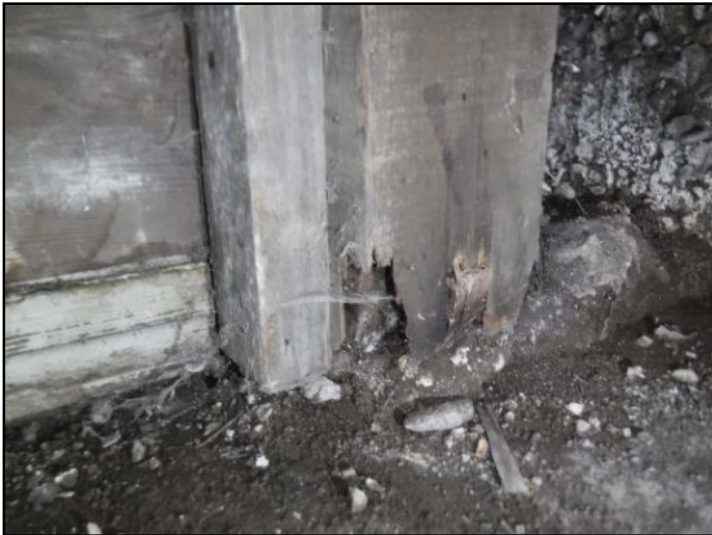
Water damage / decay noted at the base of several posts below basement stairs. Corrections by a licensed contractor is recommended.
