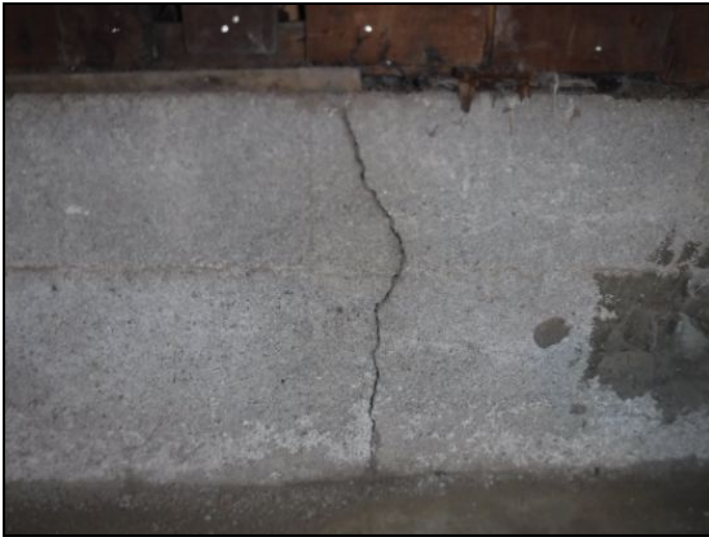
Cracks (1/4" or less) present in: foundation walls. Consider sealing them to prevent water infiltration. Generally speaking, cracks that are less than 1/4" are not commonly regarded as being structurally significant. Seal and monitor.
